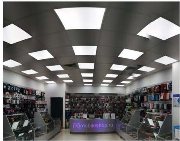
Embedded LED Panels in Russia
